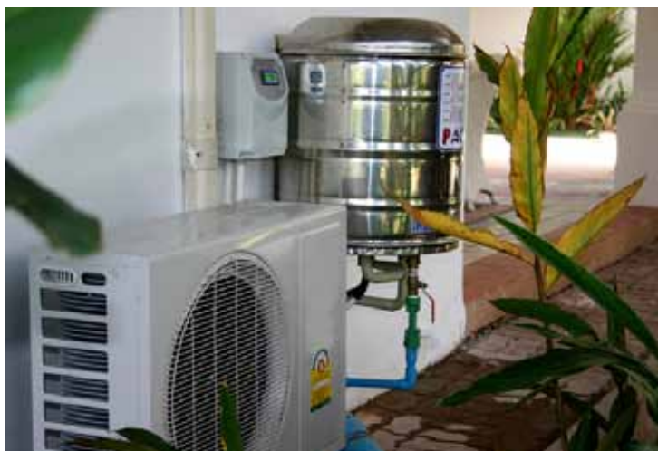
Hot water heat recycling © www.silverhawk.co.th
