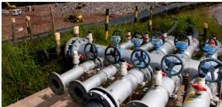
Methane recovery at landfill © Arcadis
